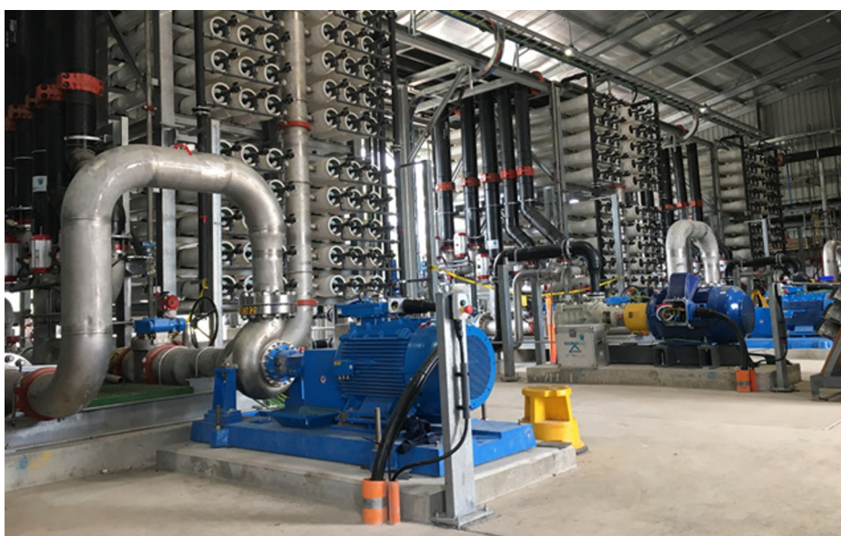
Inside the Osmoflo Brine Squeezer (OBS) plant at the Ranger mine site (photograph courtesy of Osmoflo).
