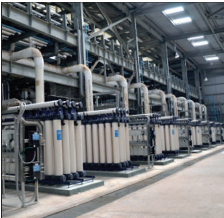
Inge GmbH played a vital role in a major project in the Indian city of Jamnagar. It supplied the ultrafiltration modules used in the pretreatment stage for reverse osmosis in the sea-water desalination process used at a refinery complex. Over 4000 T-Rack® 30 modules went online in April 2017 (photograph courtesy of Inge GmbH).
